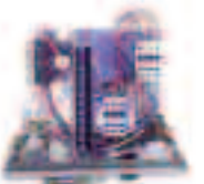
End/Booster Pump Box
